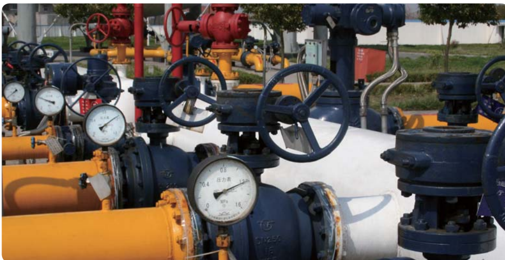
Gas meters in processing station
